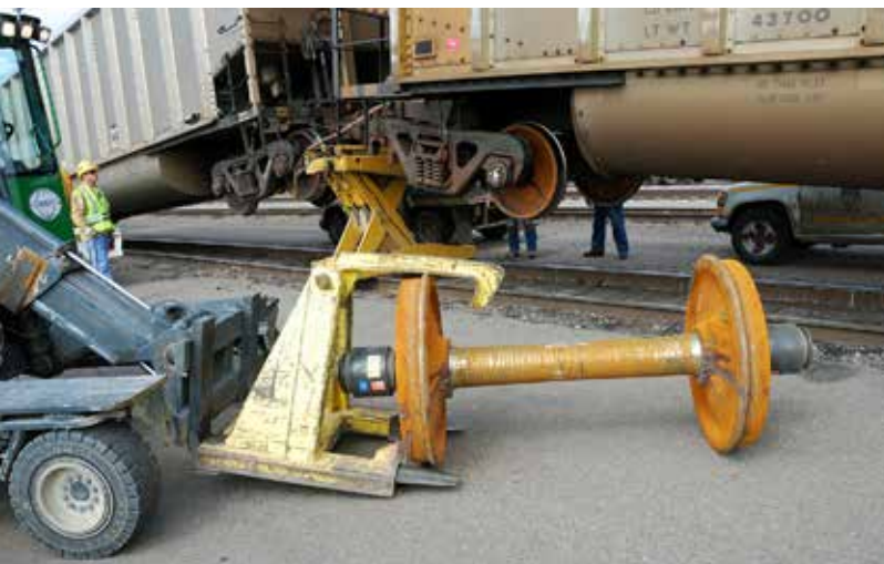
3 With the offending wheelset removed and out of the way, a crewman operating the Combilift plucks a new wheelset from a lineside flatbed truck and positions it near the car for insertion.
