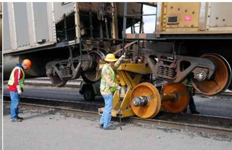
4 The new wheelset in position, workers lower the jack, guiding the car to line up the new axle with the sideframes. Total time to change the wheelset? Typically 12 to 15 minutes.
