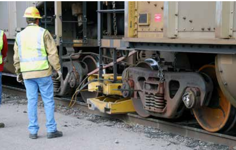
1 The first steps to changing out a bad wheelset are to insert a jack between the cars, chain the bolsters to their frames, and attach the good wheelsets to the bolsters with nylon rope.
